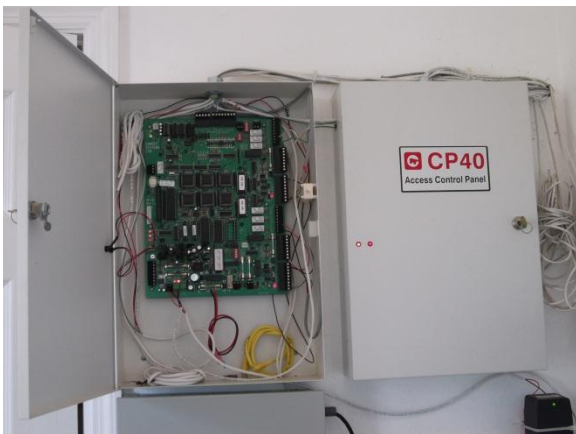
Gatehouse Access Control Panel
